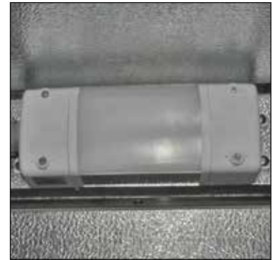
LED light fixture
